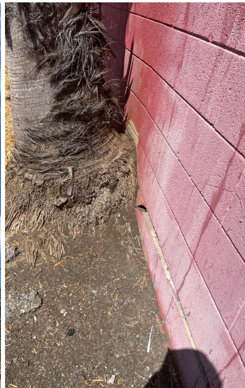
Tree pushing on the wall damaging the wall's integrity.
