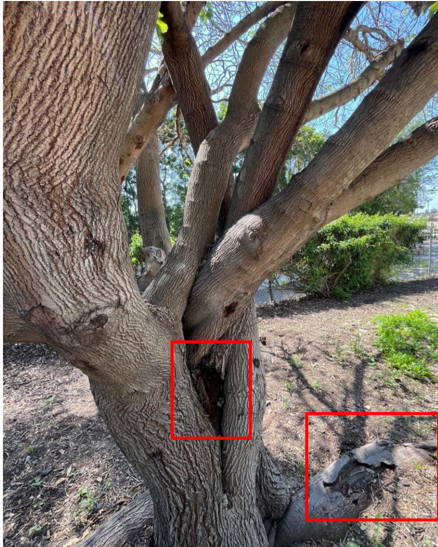
Tree has damaged roots and decay in the main joint of the trees.
