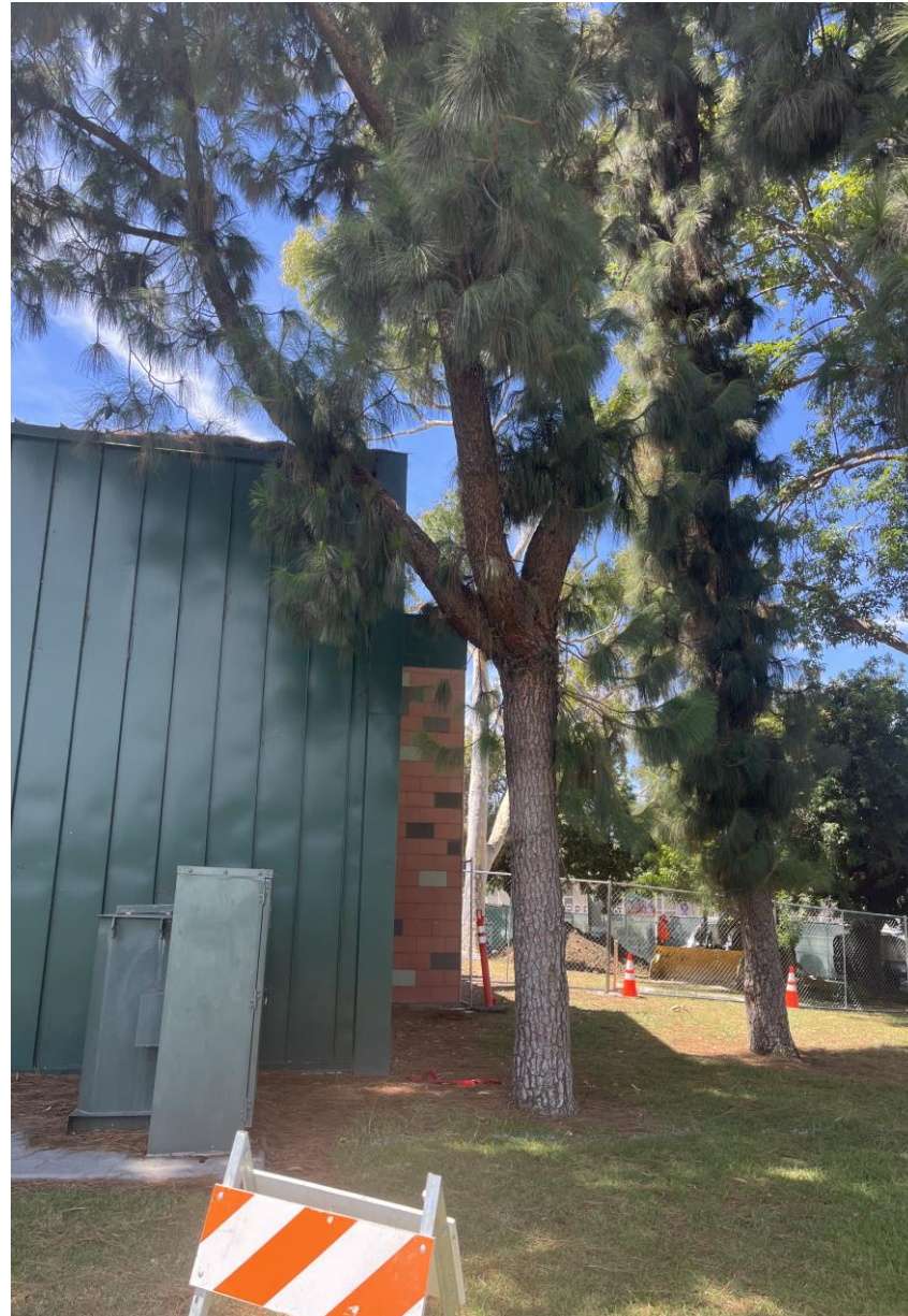
Tree needs to be removed due to violation with SCE. Too close to the transformer
