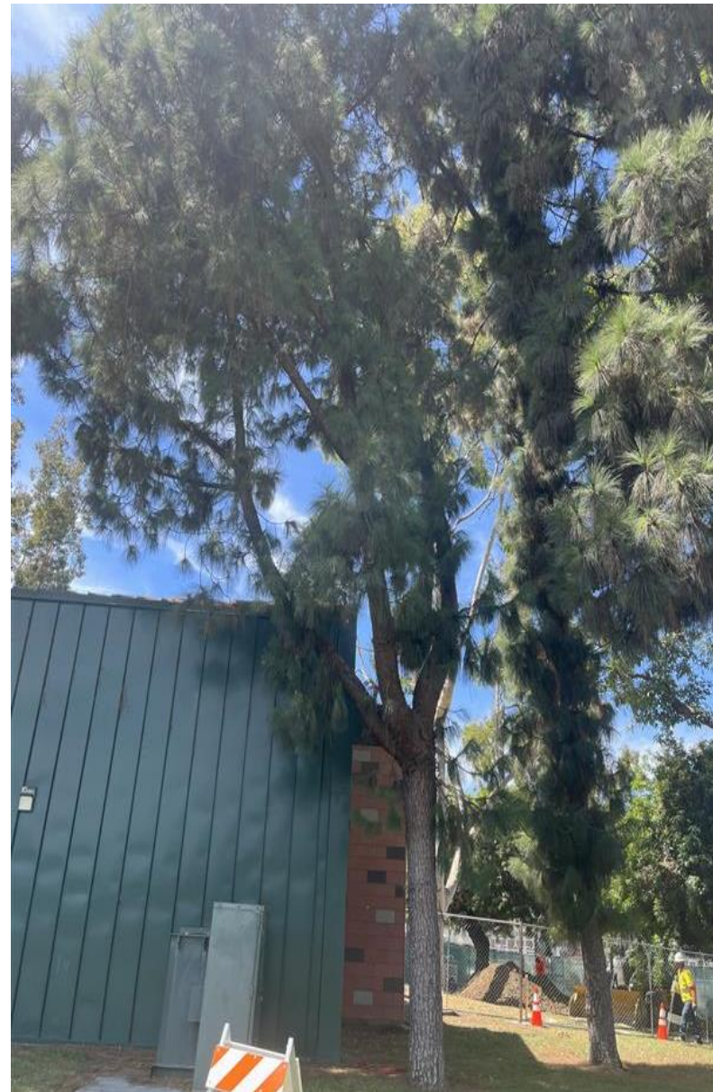
Tree needs to be removed due to violation with SCE. Too close to the transformer
