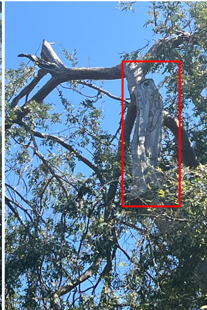
Primary Leader with an old wound. Overall weak point in the tree. Hanging over the walk path along Carson St. Corrective pruning would remove over 50% of the canopy.
