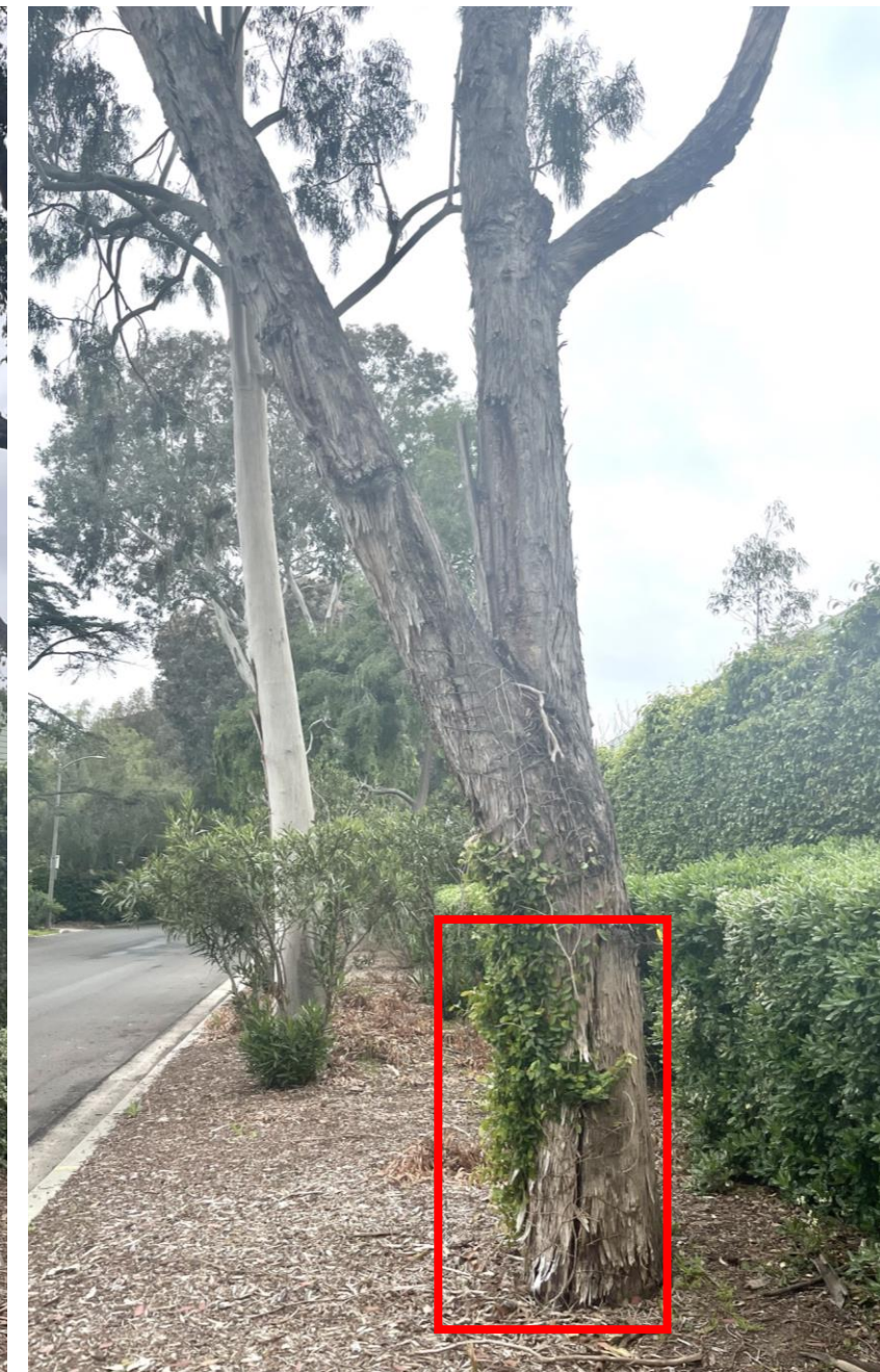
Large tree with a crack in the main trunk of the tree.
