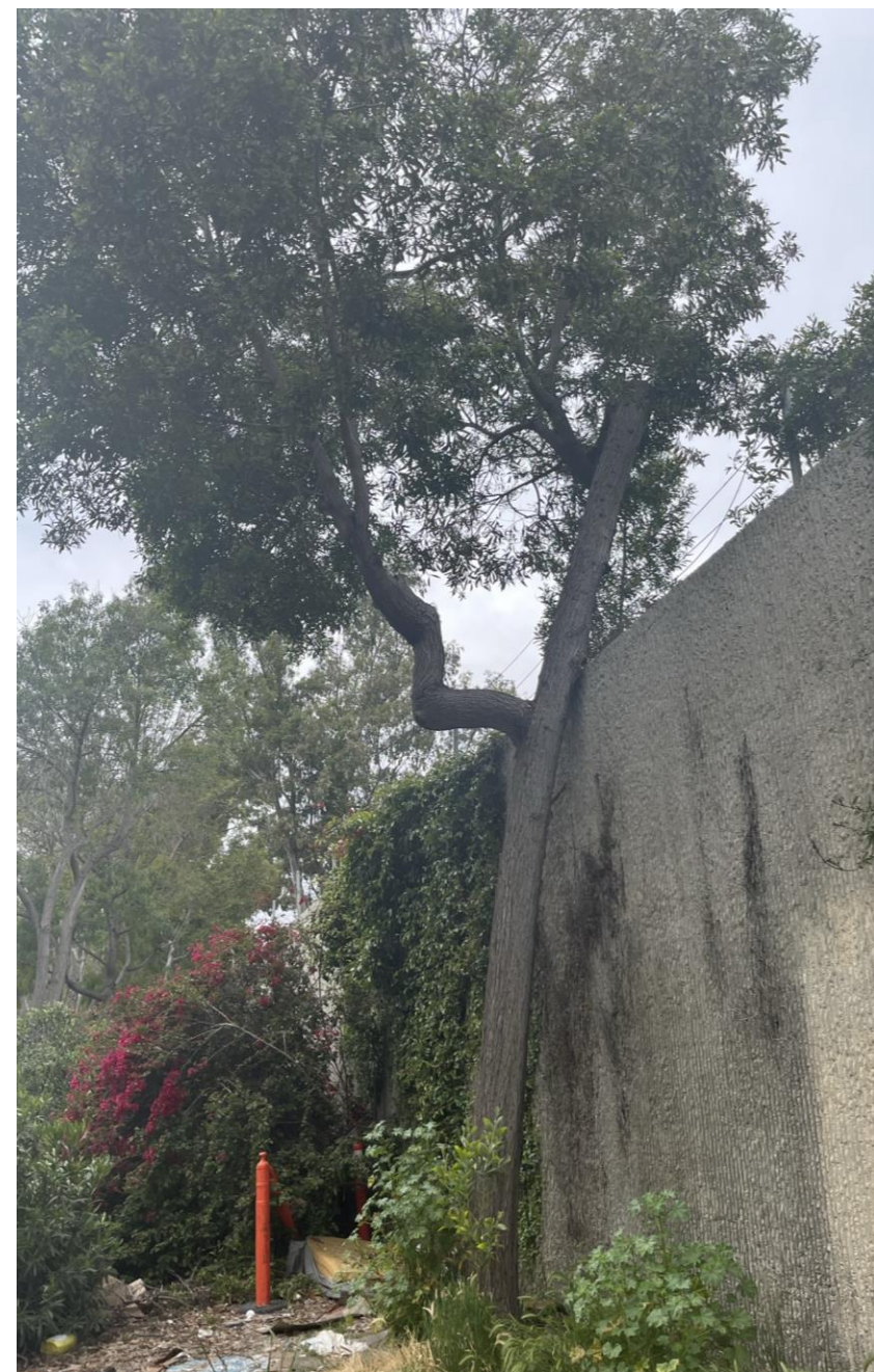
Tree is leaning on the wall of the adjacent property
