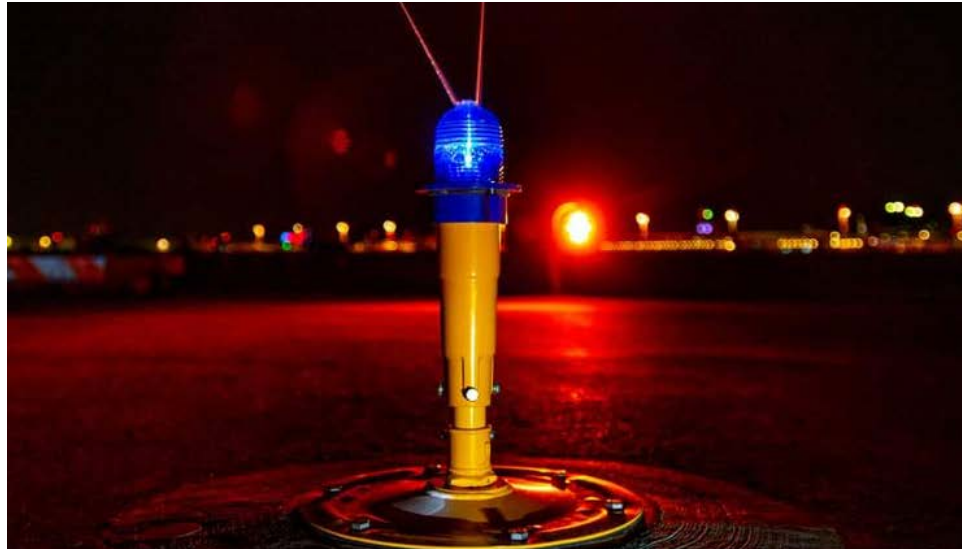
Example of new LED elevated edge lights
