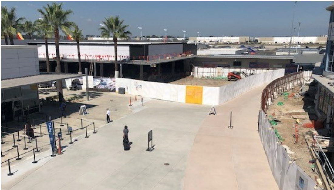
A peek behind the construction walls near the historic terminal and new Baggage Claim facility
