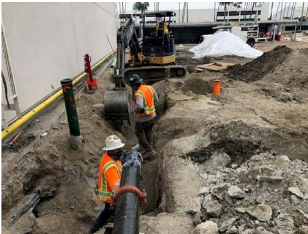
Contractors install a new water line for fire suppression adjacent to the CBIS facility footprint.
