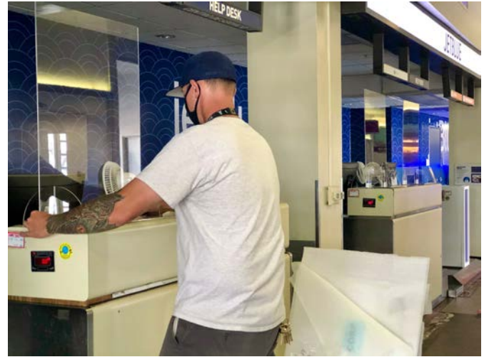
Plastic shields are installed where physical distancing is not possible.
