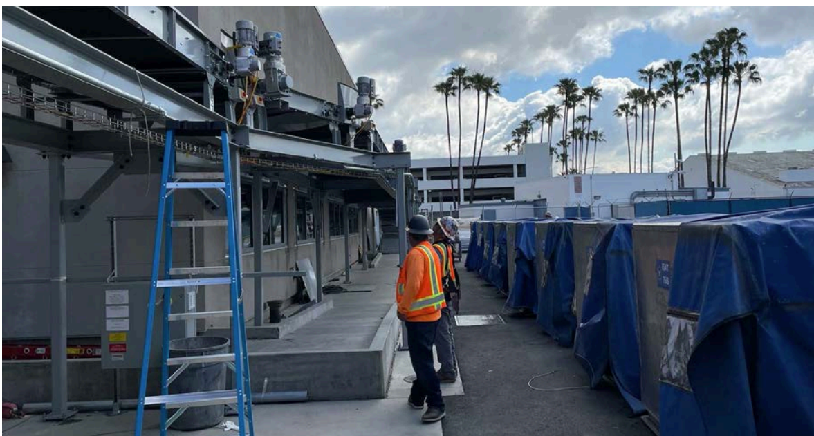
Testing of the oversized baggage system from Ticketing into the CBIS building is underway
