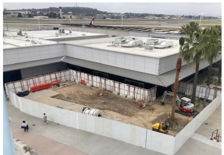
A new shade structure will be installed near the security screening checkpoint
