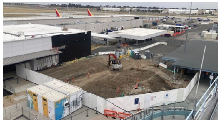
Baggage service offices and a new concession space are under construction adjacent to the new Baggage Claim facility
