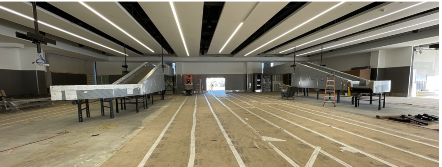
The interior of the Baggage Handling System
