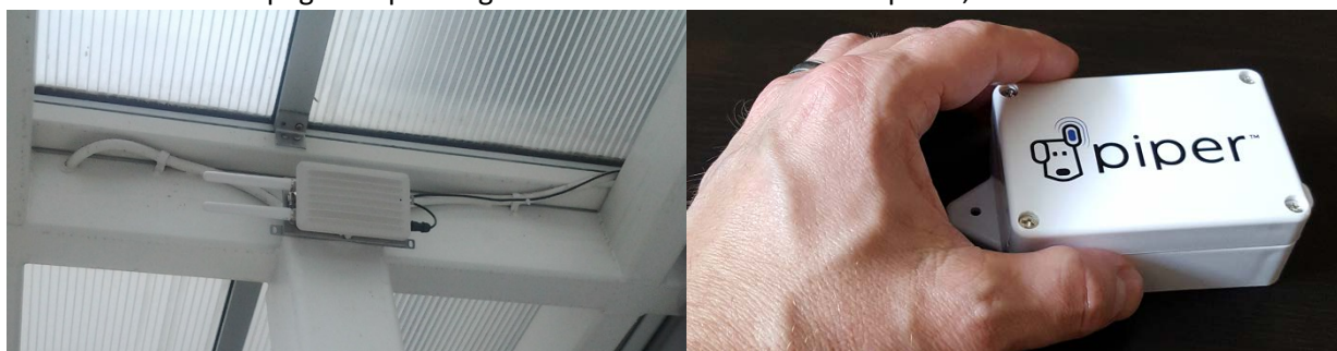
Example sensor installation
