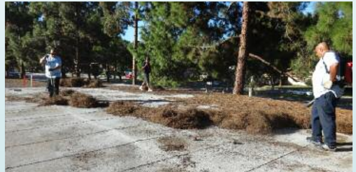
Jorge Acevedo, Everado Sanchez, and Carl Lindsay clear debris from at El Dorado Park West roof.
