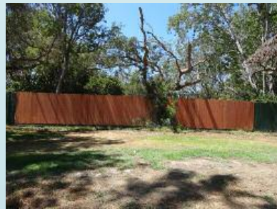
Facility Maintenance staff members Luis Oviedo and Pedro Sosa installed new fencing at El Dorado Regional Park Archery Range.
